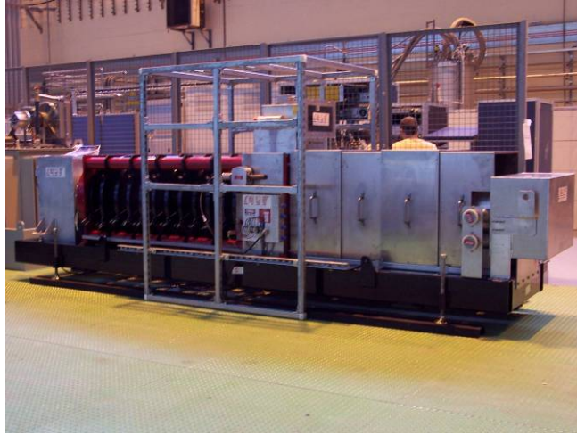
Figure 4.3.2: The klystron installed at the Saclay test stand
